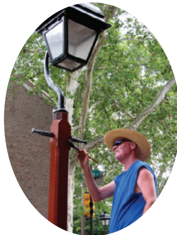
500 Franklin Lights were replaced in 2007, funded with $600,000 from a SHCA campaign. This project insured a brighter and safer neighborhood.
